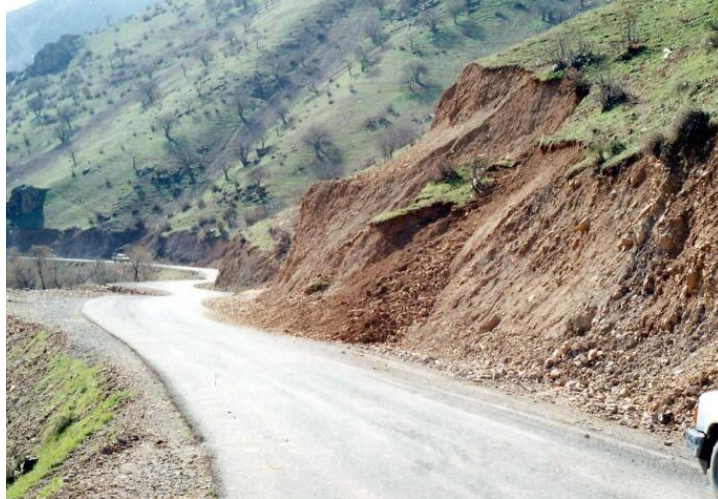
Figure 10. An example of roadside landslides on Jkr rock facies due to road excavation. The fragmented structure of the area shows a high potential for landslides. Photo from Foriab Road to the northwest.
